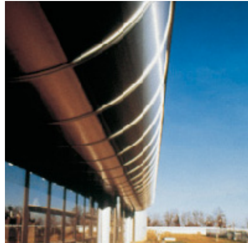
On the upper floor, the rainwater drainage is concealed behind the stainless steel cladding.
